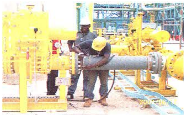
NDES staff carrying out radiographic inspection on the West Africa Gas Pipeline at the Takoradi Thermal Power Plant.
